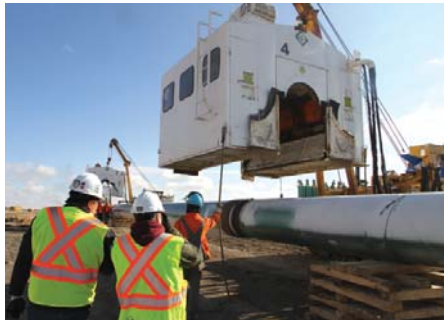
A welding shack is lifted into place over one of the weld spots.
