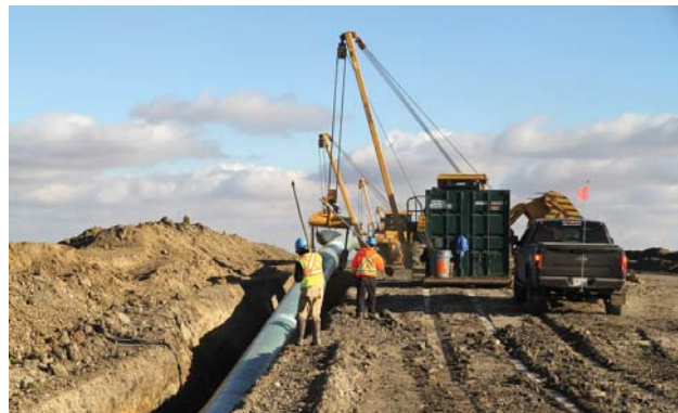
Workers watch for rocks and debris in the trench as the pipe is laid in.
