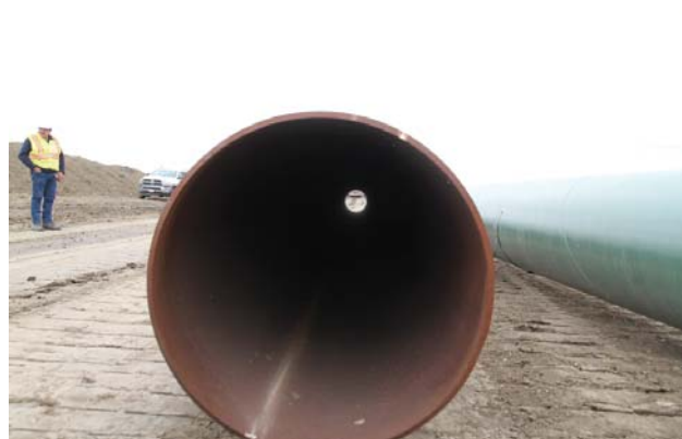
Pipe laid out on the right of way before bending and welding.
