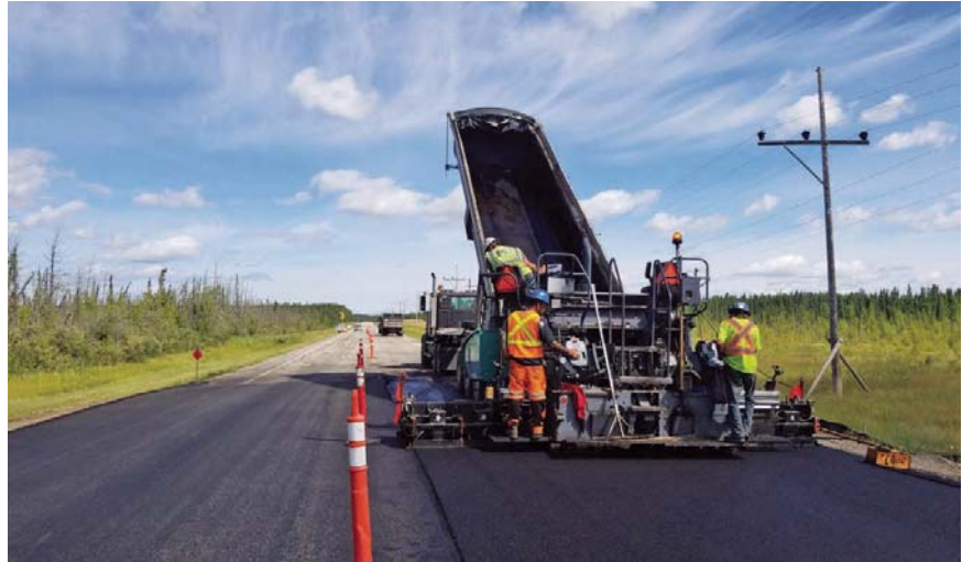
Saskatchewan Highways has released its fall tender schedule, with $437.4 million worth of work, including repaving of Highways 8 and 308 in the Rocanville-Welwyn area and the addition of passing lanes on Highway 16 from Yorkton to the Manitoba border.
