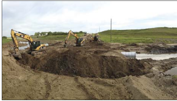
This photo was taken in the RM of Wallace, where the flooding damaged 211 roads. Since then, 205 of them have been fully repaired, and DFA funding will cover the costs, which the RM estimates are near $1 million.
