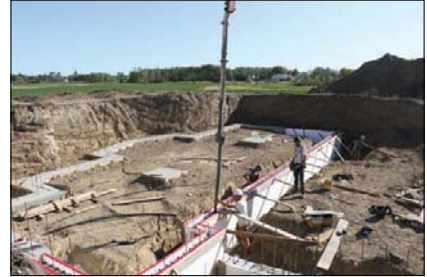
The concrete pour for a basement for a new home that is being built in Brylee Estates.
