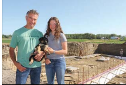
Darcy Borys, the owner of Brylee Developments, his daughter Levi, and their new puppy Duster. In back is the basement of a new home being constructed in Brylee Estates.
