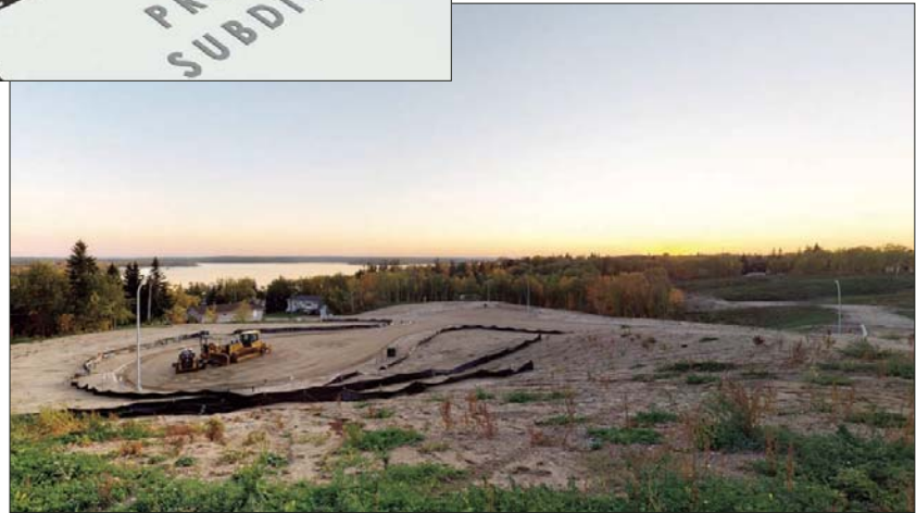
Right: Development of the new subdivision in Kenosee Lake. The lots are ready fore building and fully serviced.
