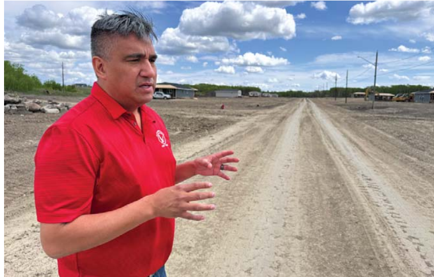
Chief Evan Taypotat looks over a new housing development under construction on Kahkewistahaw First Nation.
