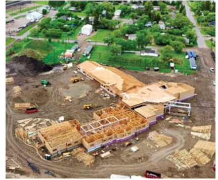
Construction progress on the new 33-bed long term care facility in Grenfell!
