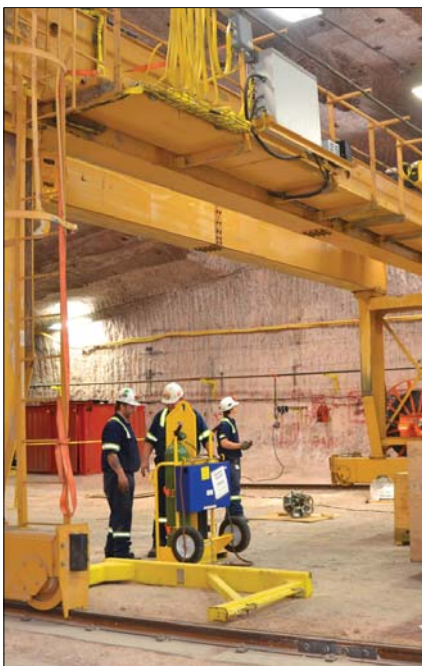
K2 shop gantry crane: The K2 four-rotor miner assembly shop was built beginning in November, 2009, to facilitate the assembly of two new four-rotor miners.
