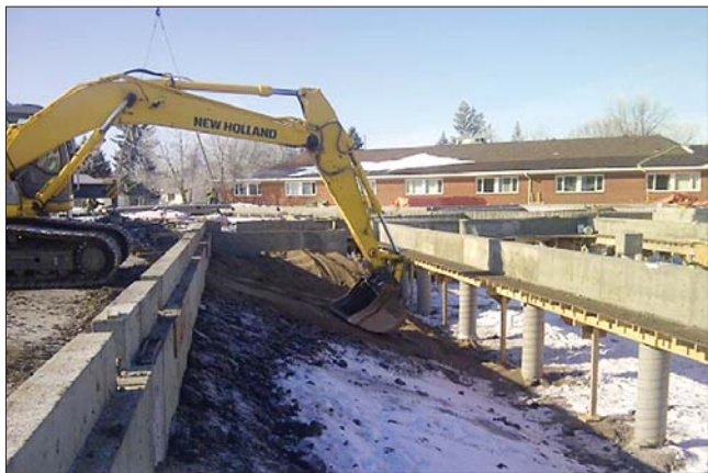
Progress on the long-term care addition to the Redvers Health Centre as of March 2012.
