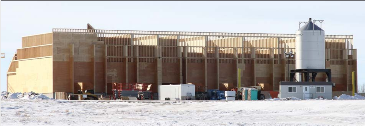
Work continues on the new fertilizer shed at Parrish and Heimbecker just west of Moosomin. The new dry fertilizer facility will be 35,000 square feet when finished. A liquid fertilizer facility is also being added at P&H's facility at Moosomin. Six 300 metric tonne tanks will be installed.
