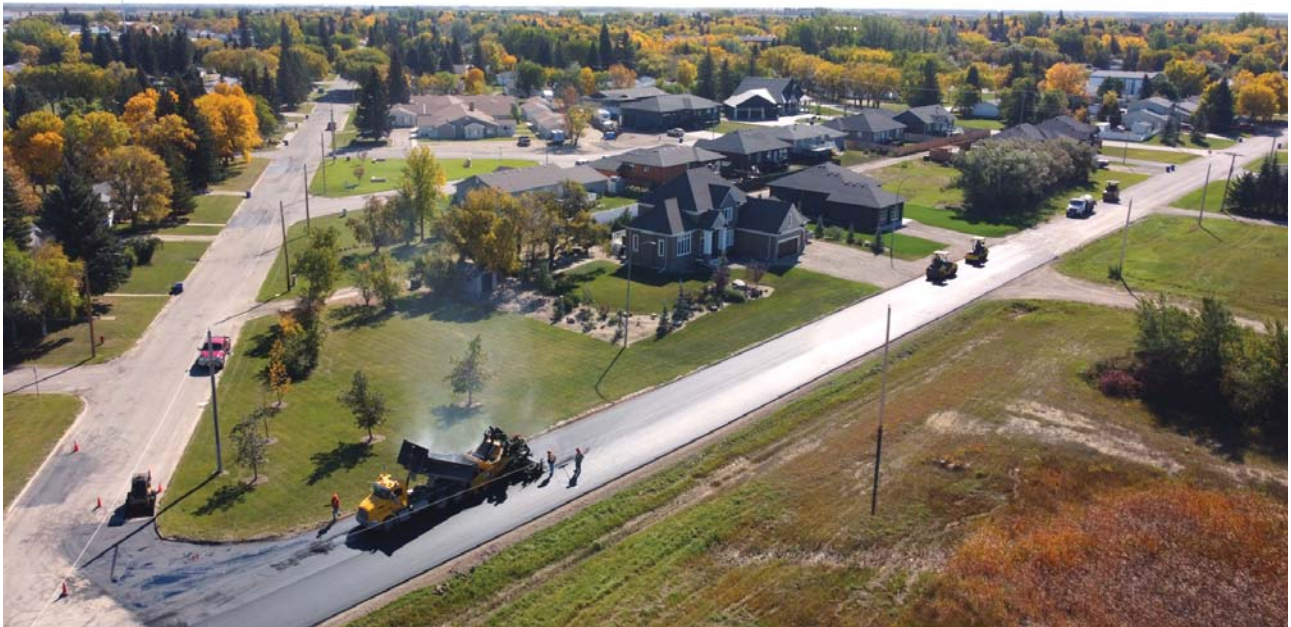
The town of Moosomin has been doing a lot of paving this fall. Here a paving crew works on paving Cook Road.
