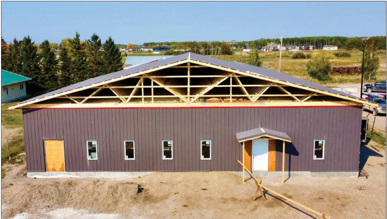
The 5,600-square-foot expansion on the front of Bumper to Bumper in Rocanville.
